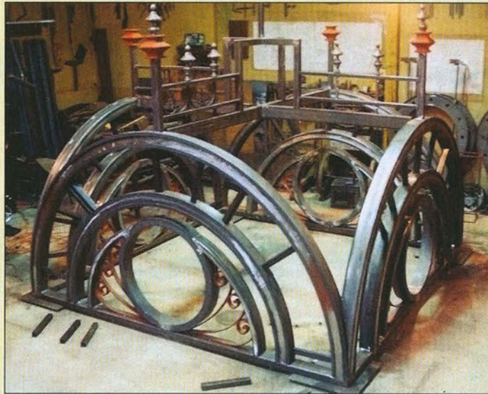
Top Frame Structure. Fabrication of the upper frame joining the columns with the clock face required structural welding on all six sides.
