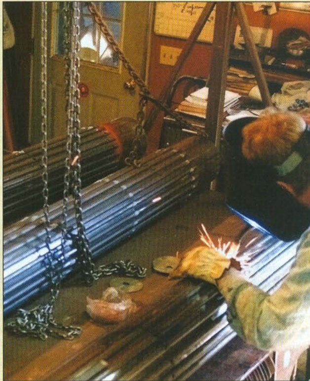
Welding Flutes on Columns. 288 reeds cut from \frac{3}{4} -inch, half-round steel were plug welded on the pipe columns.
