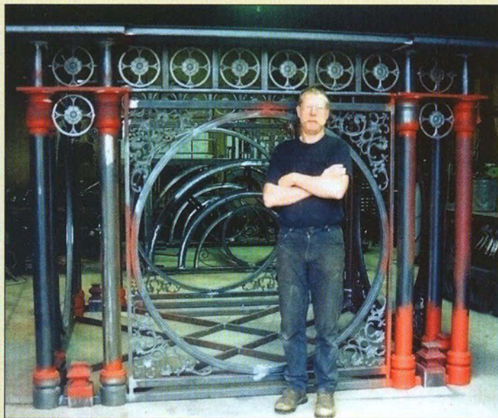
Lee Badger with face frame. Each of the tower's 10-foot x 10-foot frame sections was completed individually, wiped clean with denatured alcohol, pre-primed with high-build auto-body primer, and "finished" with a protective working coat of satin black enamel.
