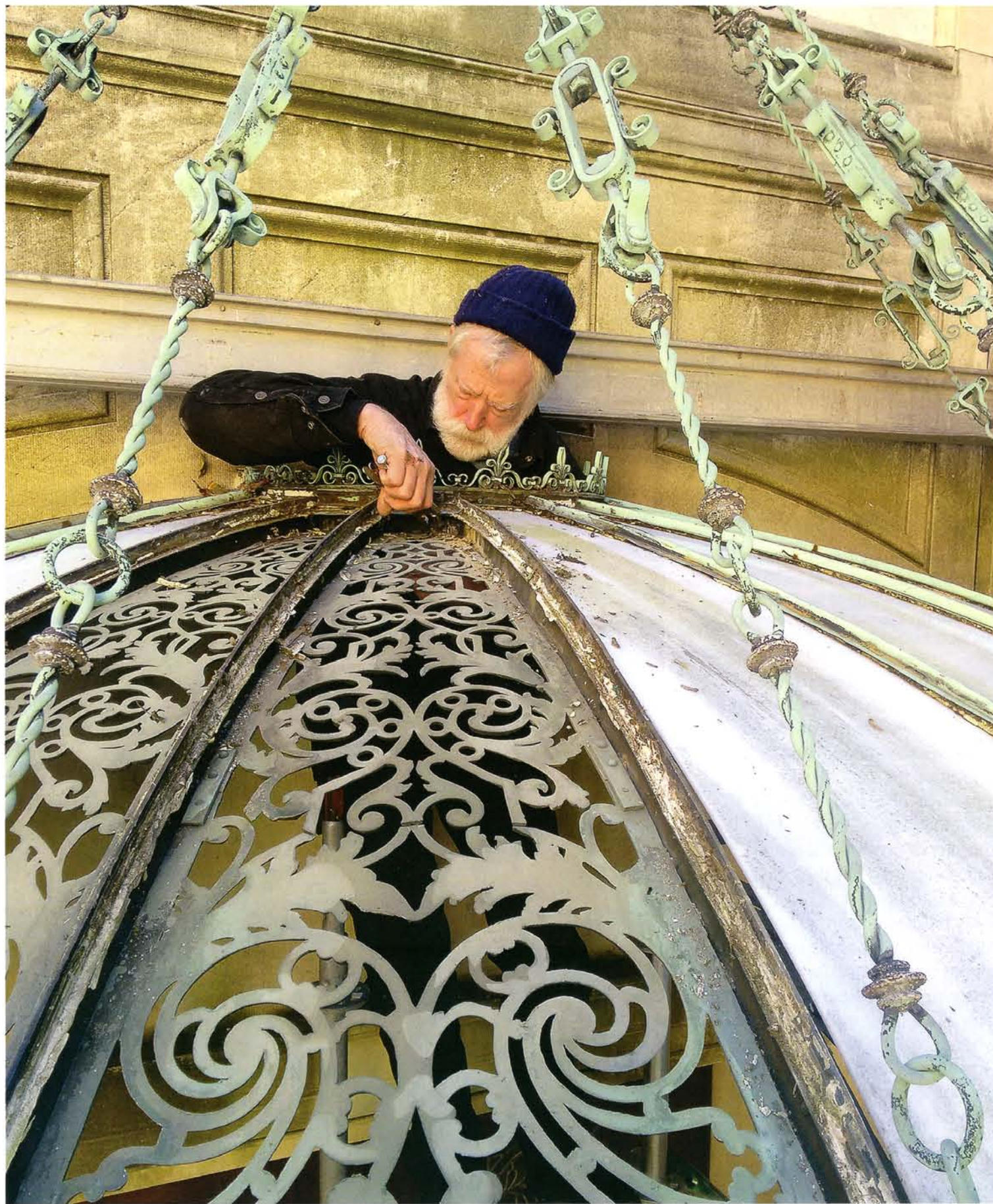
Above: Restoring an ornate entrance canopy created by Tiffany Studios in 1905 on the Evergreen Museum and Library, a Johns Hopkins University Museum in Baltimore, MD.
